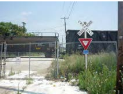
Disconnected roadway due to rail crossings
